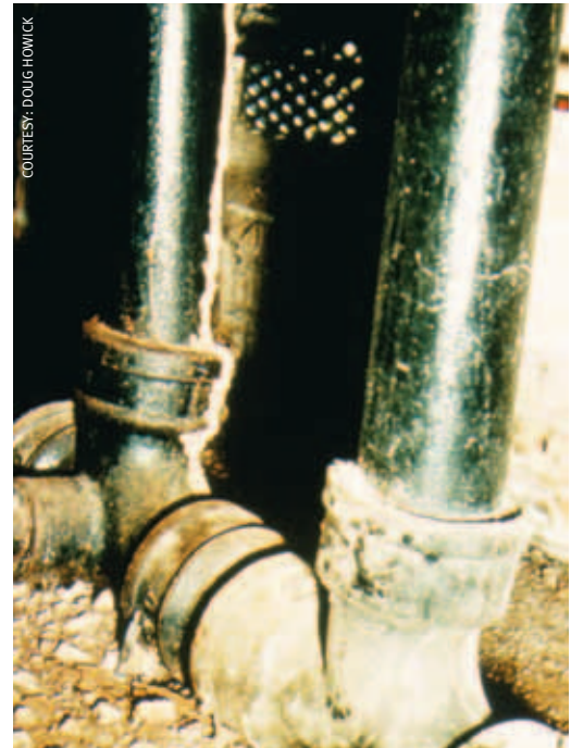
Mud shelter tubes over subfloor piping are signs of termite activity.
