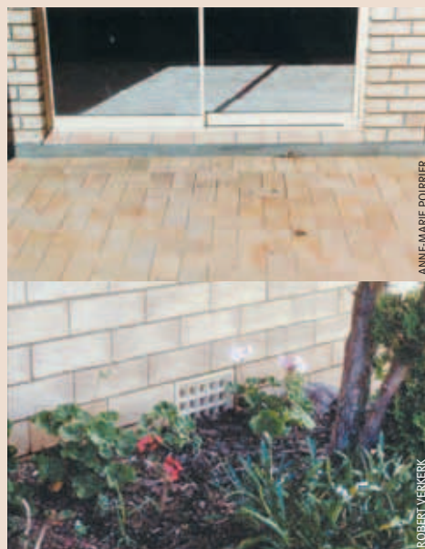
An exposed concrete slab, like the one in the top photo, acts as a physical barrier that will bring termite activity into the open. If it's covered with shrubs and plants, as in the photo below, termites can gain concealed access to structural timbers.
